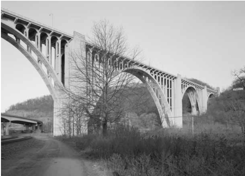
George Westinghouse Bridge, Spanning Turtle Creek at Lincoln Highway (US Route 30), East Pittsburgh, Pennsylvania, c. 1968.
